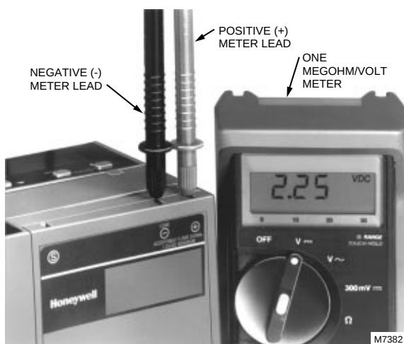
Fig. 16. Flame signal measurement.
